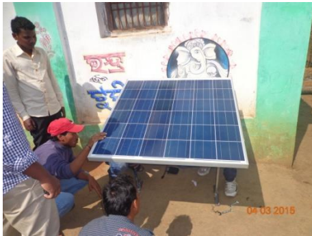
Solar Panel powering the inverter
