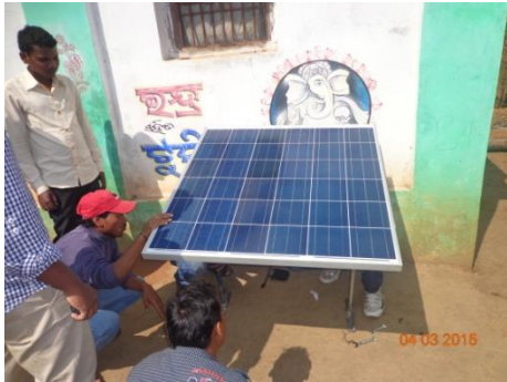
Solar Panel powering the inverter
